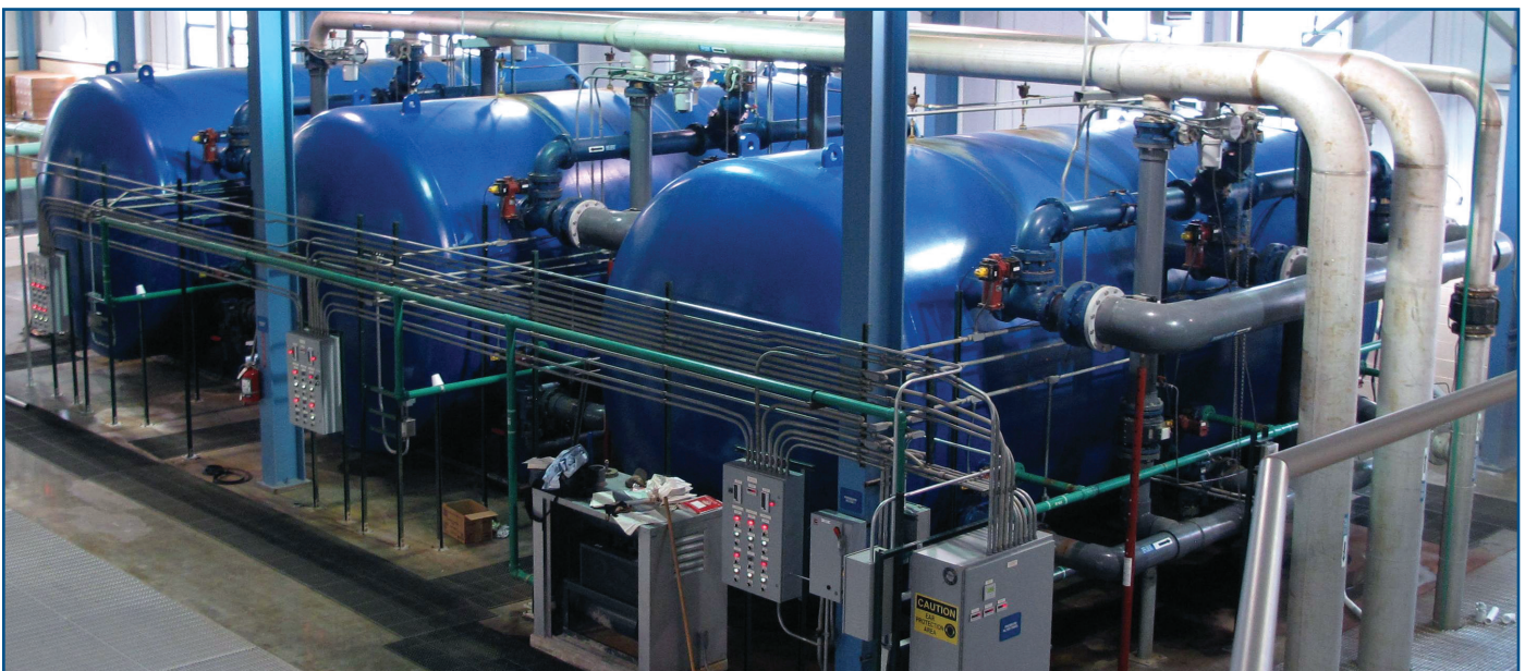
GreensandPlus Pretreatment for RO Filter System 4.2MGD
