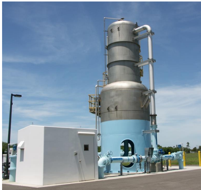
Vacuum Degasifier with I&C Building
