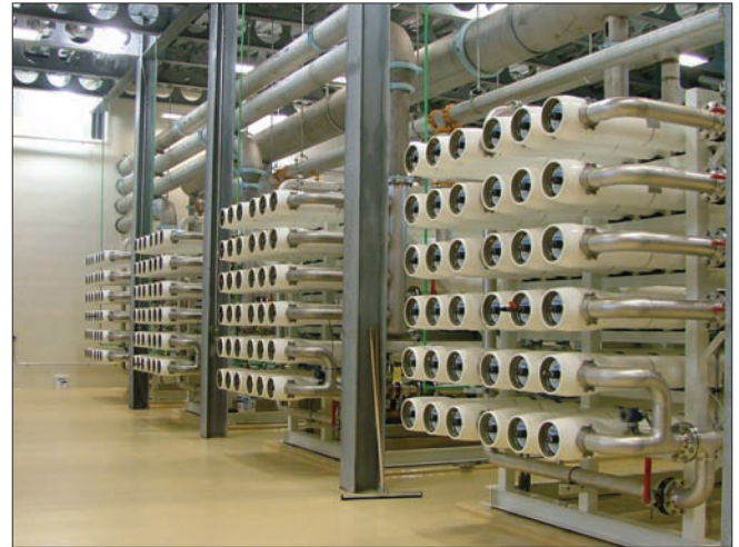
The Hydranautics RO membrane system consists of four skids. Each skid contains 36 tubes with 252 individual membranes. The four skids therefore, have a total of 1,008 eight-inch diameter membranes. The membranes are two stage units.
