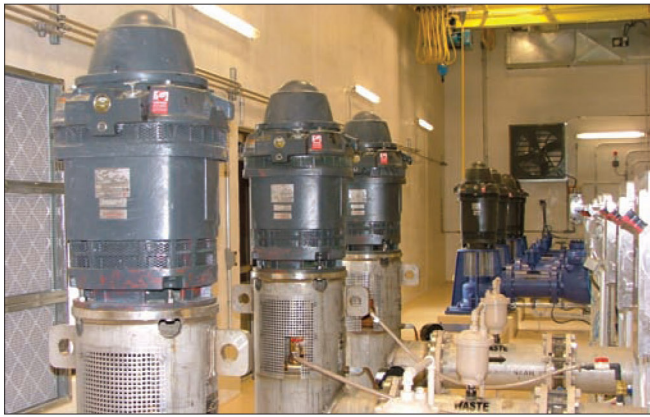
This photo shows two sets of pumps; the nearest pumps with tan piping transfer concentrated reject water to disposal wells. The pumps in the background are the four raw water pumps on variable frequency drives (VFDs).
