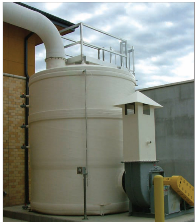
This photo shows the scrubber treatment equipment used to handle the accidental release of chlorine gas. This equipment is usually designed to neutralize and absorb the entire contents of a one-ton cylinder. Please check out the article "Containment systems help ensure chlorine capture" by Gary Armentrout in the July 2004 issue of The Kansas Lifeline magazine for more information on this subject.
