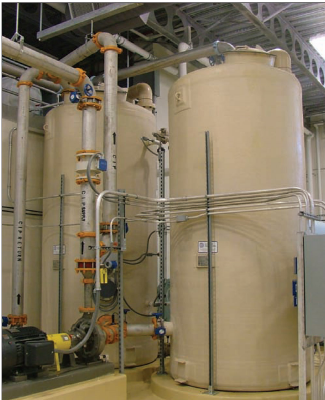
This tank and pump arrangement is the clean-in-place system which uses RO treated water for cleaning the membranes.
