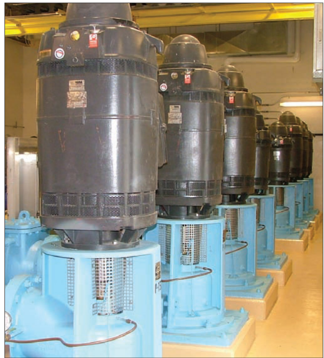
Six of the eight pumps shown here pump treated water to the distribution system. The two pumps in the center of the row are pressure filter backwash pumps.
