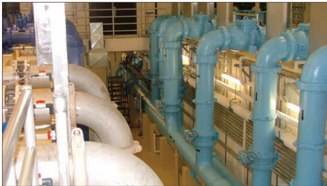
This is a shot of the pump and piping gallery with waste and raw pumps on the left and finished water and pressure filter backwash pumps on the right.
